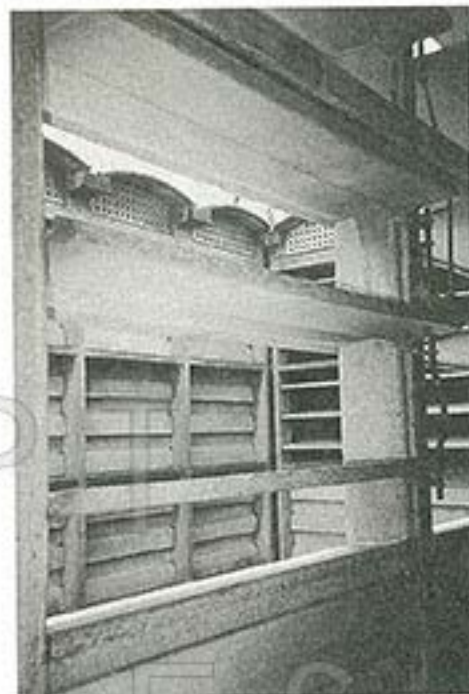
The hand operated asbestos-cement louvres
